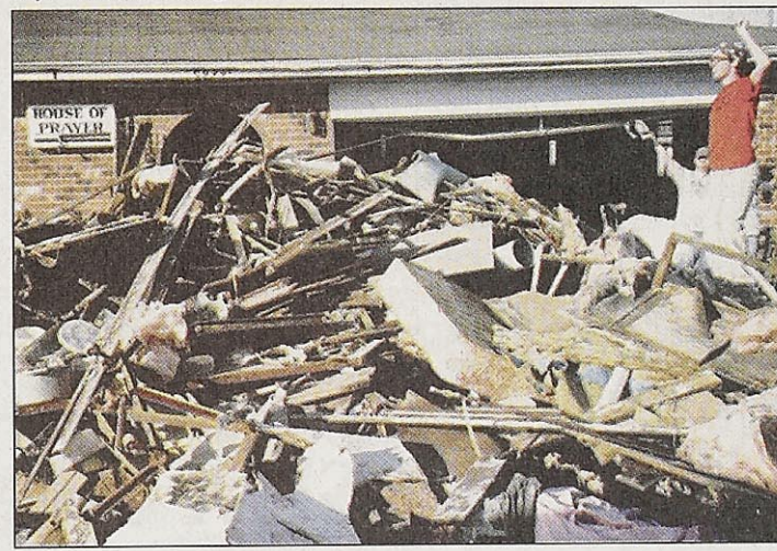
BELOW: Geoff Stewart, a junior at St. Louis Community College-Forest Park, climbs on top of a debris pile and raises his fist in triumph at the end of a long day. Stewart's team gutted a church in the Ninth Ward.
