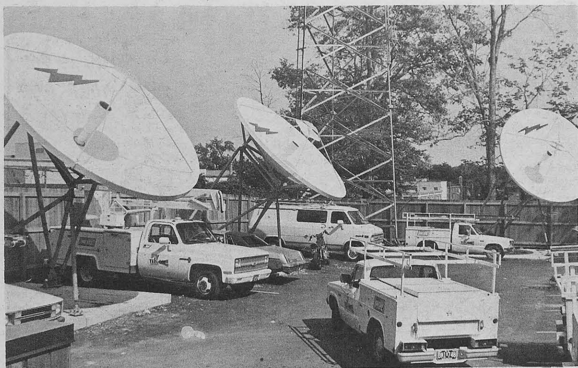
Receiving dishes are the most visible cable TV equipment. These are located at Telcom's Kirkwood office. photo by Brian Schaff
