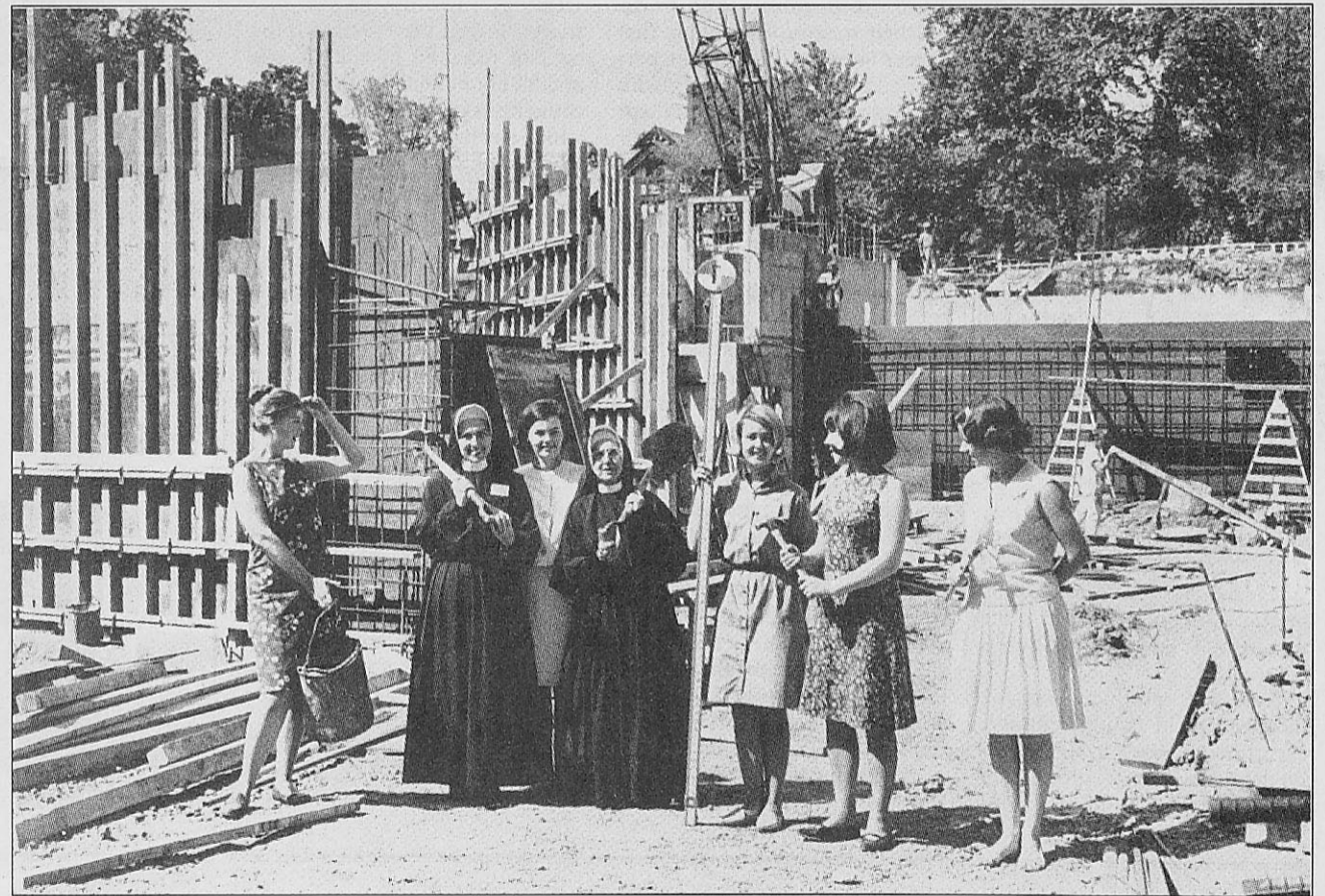
A group of Webster students and faculty stand in front of the Loretto Hilton Center construction site in 1965.
