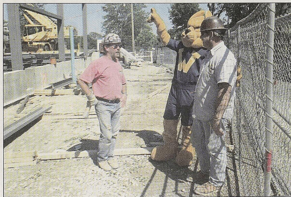
(Above) 1:14 P.M. Community Music School construction grounds. To earn a couple bucks, the Gorlok took a job as a construction foreman. Here he/she shows two ironworkers, Pete Bush (left) and Mike Blomberg, where he/she thinks the 85 foot, foam-posite bust of wacky Webster professor Lawrence Baden, should go. A brief dispute, followed by the Gorlok doing his famed "Pete's wife impression," leads to the Gorlok suffering his second beating of the day.
