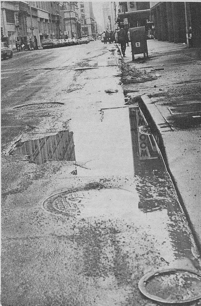
After snows disappear, potholes appear — causing more problems for cars, trucks and people who don't want wet feet.
