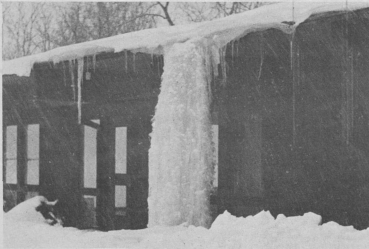
Early last week this cascade of ice was an intriguing growth on the east side of the Big Bend Building until it threatened to fall on a blue Nova. After being unable to locate the car's owner, the maintenance department used a truck, ropes and chairs to fell the sculpture. photo by Fred Luna
